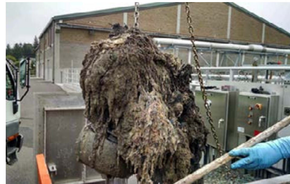
Debris wad at the waste water treatment plant.
