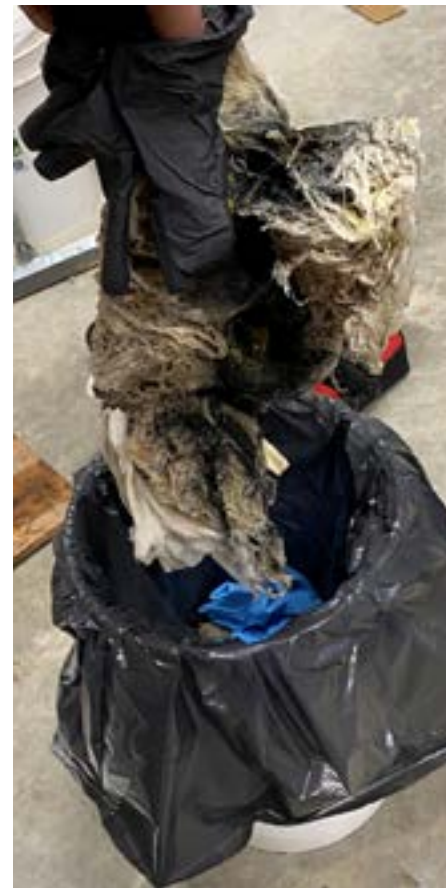
Accumulation of gloves, wipes and masks at the sewage pumping station.
